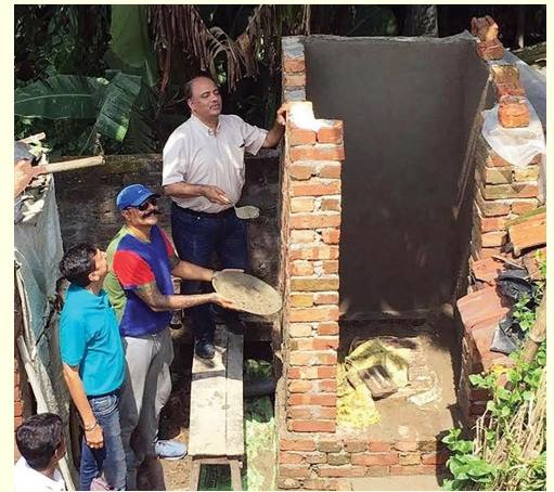
Mehta's club has constructed some 7,000 toilets in villages where people don't have toilets in their homes; here, he and fellow members (from left) Pranay Agarwal and Sandeep Shah help build one .
